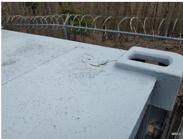
Roof needs maintenance.
