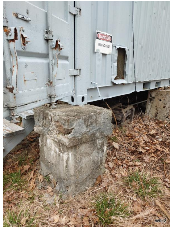
Piling deterioration, SE corner. Door cam locking levers ready to break at the welds. Brush growth inside the fence now requires bow saw to cut 7 years of seedling growth.
