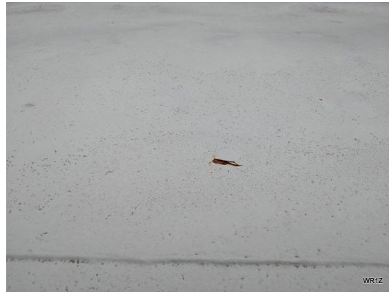
Rust spot that will perforate the roof.
