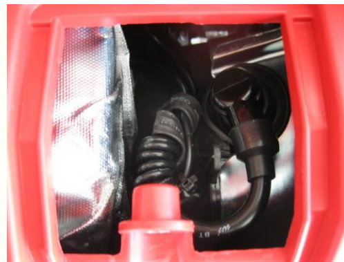
Induction pick-up wire on spark plug wire
