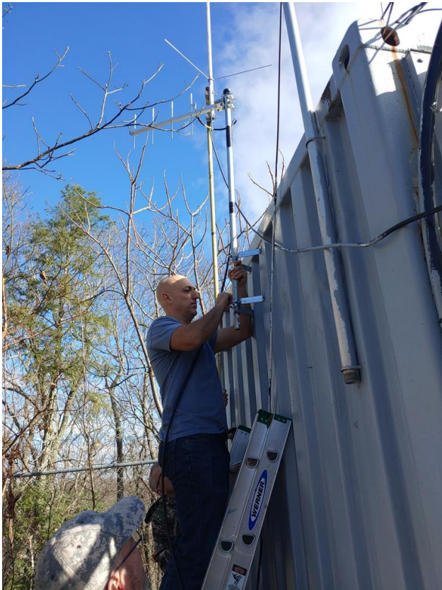
Massimo Delessandro – KC1OSQ installing the 440 FM link antenna to the side of the repeater equipment container during a recent repeater work session.
