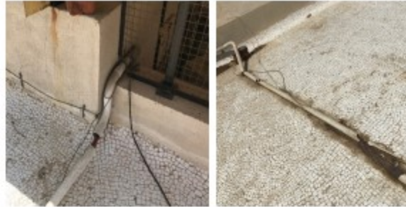
Incorrect - Conduits are damaged
