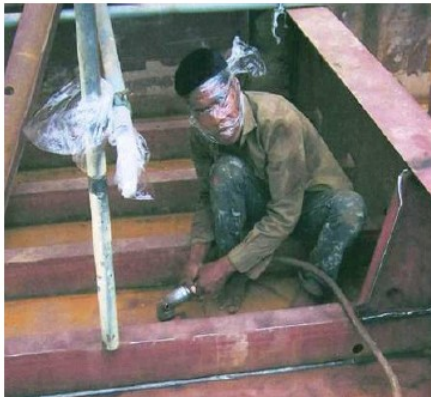
Incorrect practice - Without face shield
