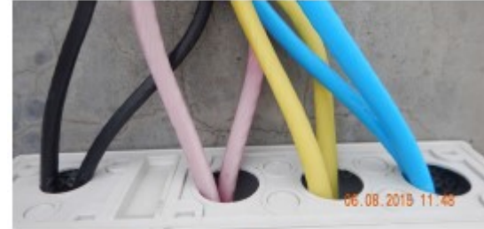
Incorrect - Cable conduit are not closed
