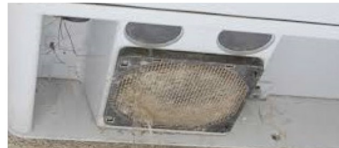
Dust accumulation on Inverter
