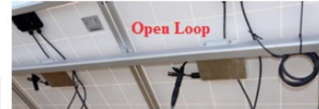
Incorrect cables connection looped loosely
