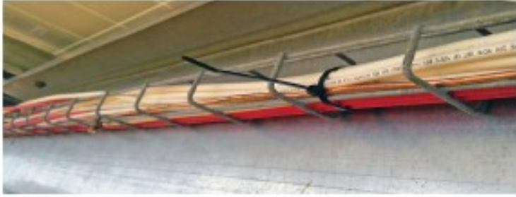
Cables are tied using cable tie
