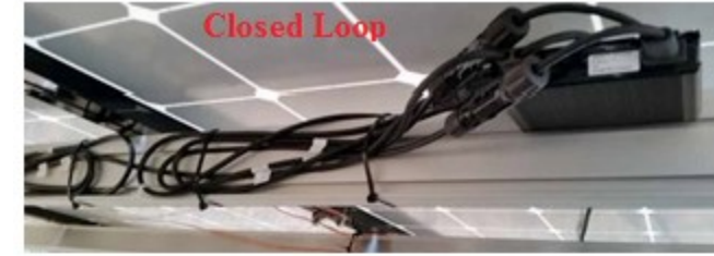
Incorrect cables connection looped tightly
