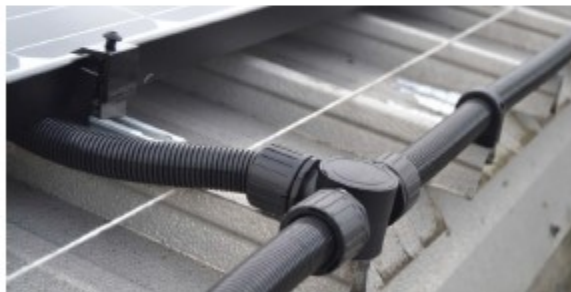
Correct - Conduits are in proper condition
