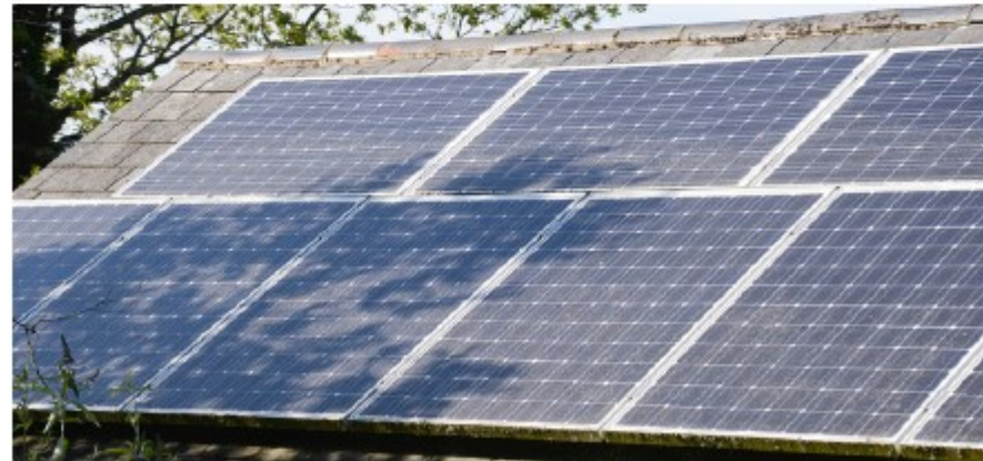
Shading on PV modules due to surrounding objects
