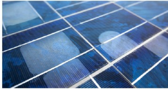
Tiny Hairline Cracks
