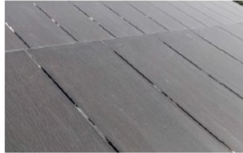
Cleaning Required Shortly (No significant financial impact)
