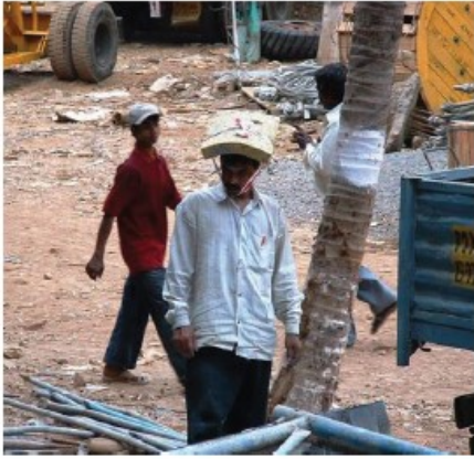
Incorrect practice - Without safety helmet
