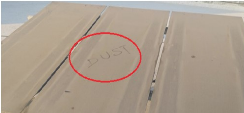
Cleaning required (Significant financial impact)
