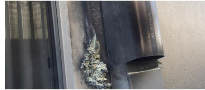
Figure 81: Inverter damage - Burn out
