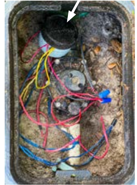
Temporary battery timer
