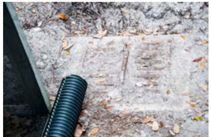
Uncovered drain packed with sand
