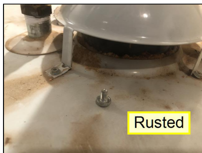
Top of water heater
