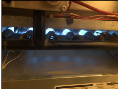
Gas furnace fire up
