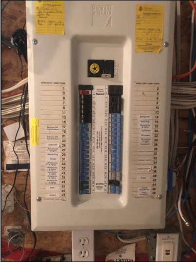
Main service panel
