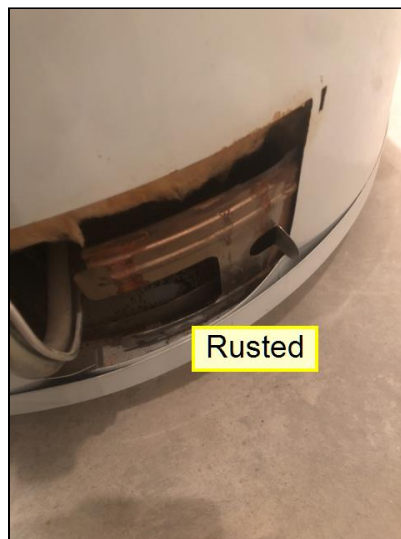
Bottom of water heater
