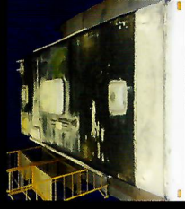
Before picture of a badly deteriorated EPDM roof.
