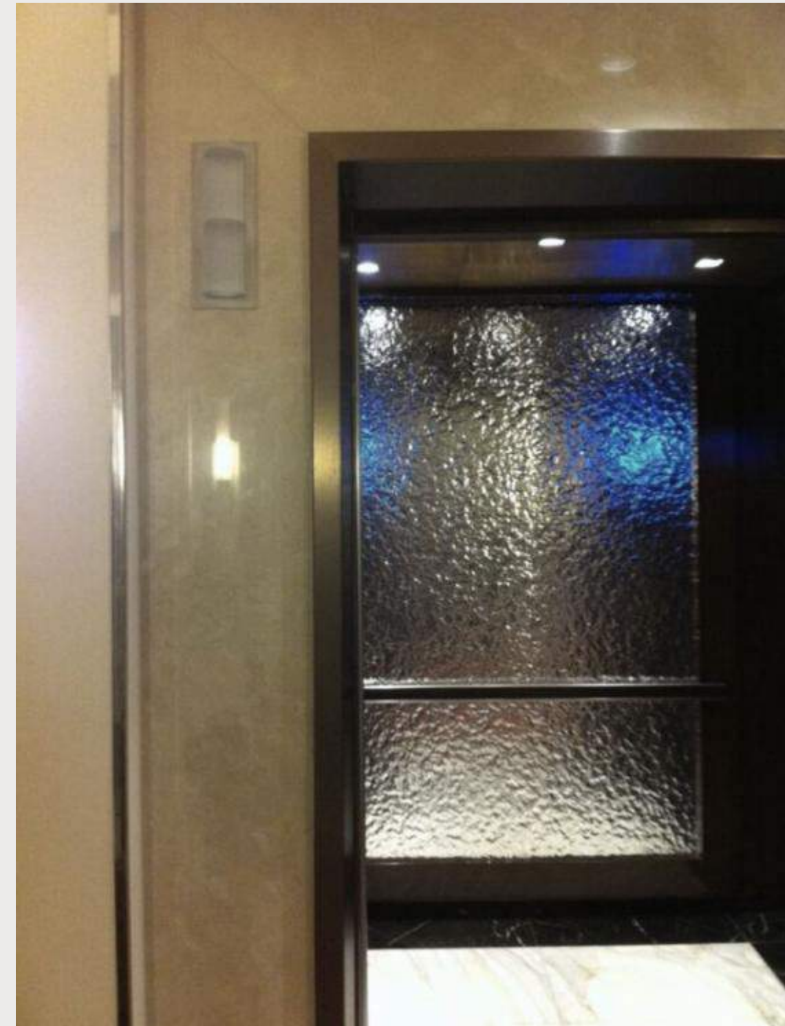
LIFT CAB INTERIOR
