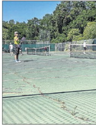
Cracks run through the tennis/pickleball courts at Larson Park in the Springs.
