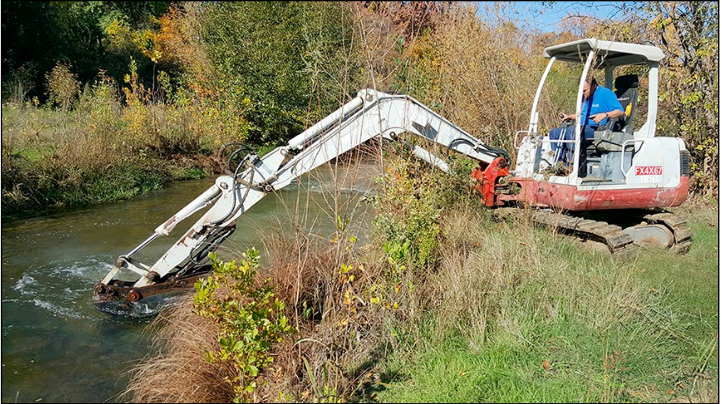
Scarification process prior to the 2016 salmon spawning season. Using expert operators, riparian damage is minimal. A biologist is always on-site before and during the process to watch for wildlife. Image Ken W. Davis.
