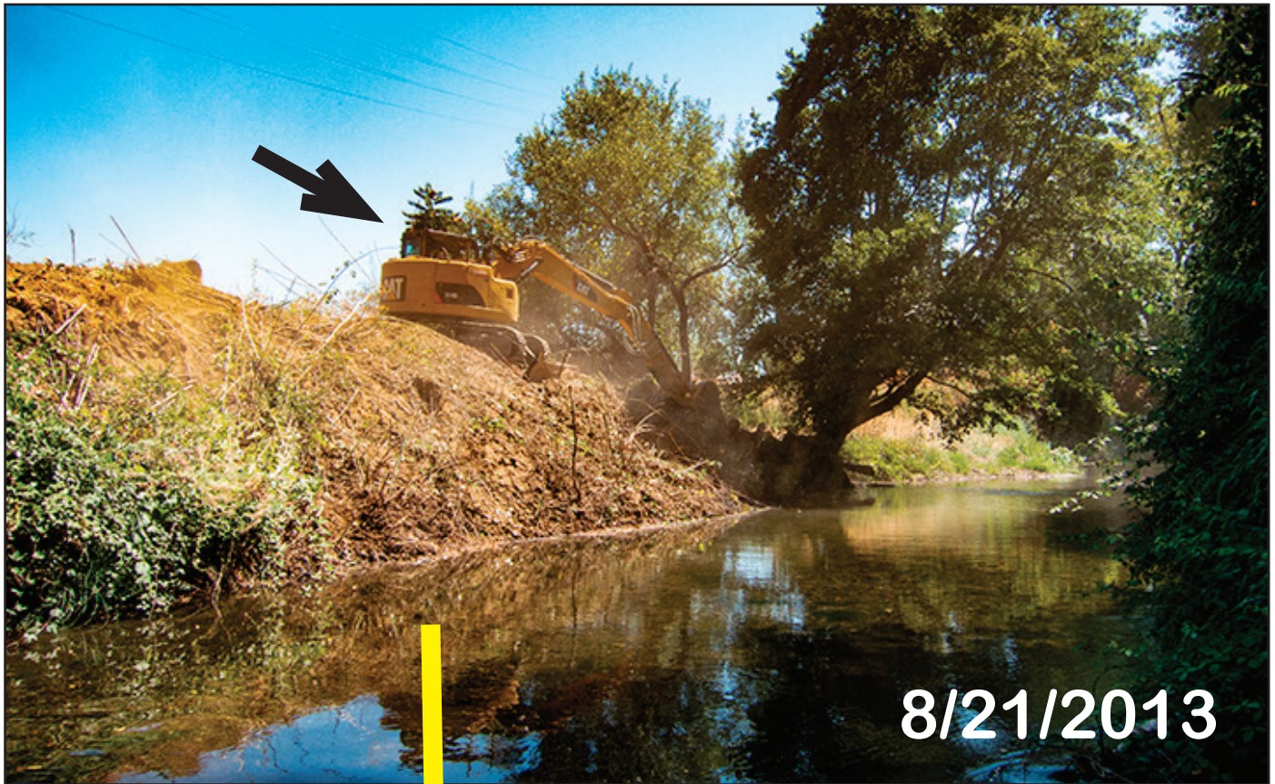
Image August 21, 2013: Shows excavator working to lower the south bank of Lower Putah Creek to create a functional flood plain. This section did not have appropriate spawning areas prior to the NAWCA 2 project and scarification. Ken W. Davis image.
