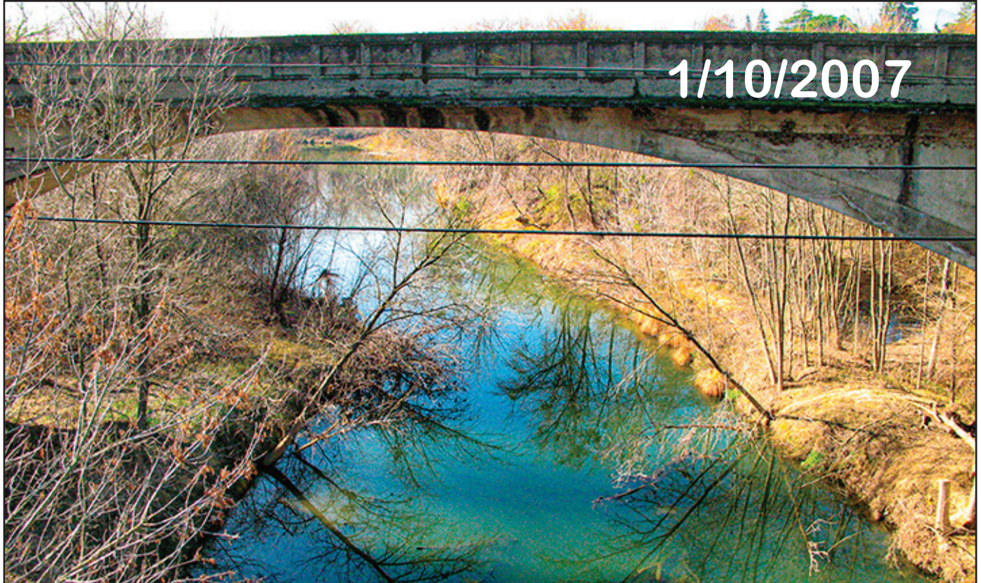
Winters Car Bridge: 1/10/2007: Image from the Winters bike bridge facing upstream with the original Winters car bridge in the image. This is an example of the “Accord” water flowing through an area that is distinctly poor habitat for salmonids and aquatic biota. Ken W. Davis image
