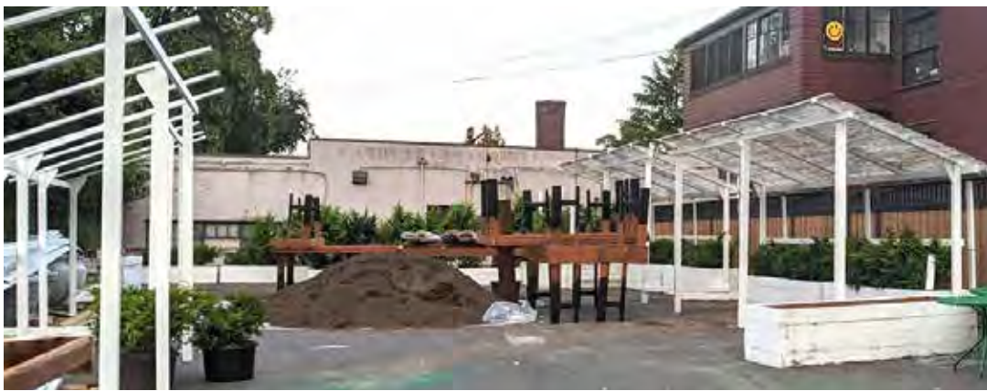
Patio construction began last summer. Semi-enclosed dining rooms surround a central bar.
