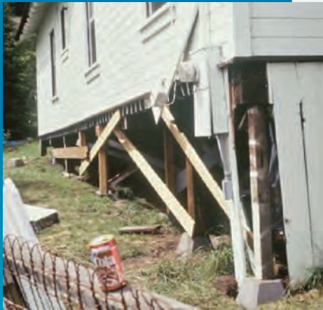
This home's pier-and-post foundation was damaged during an earthquake. The diagonal bracing was added after the earthquake to temporarily stabilize the home during repairs.
