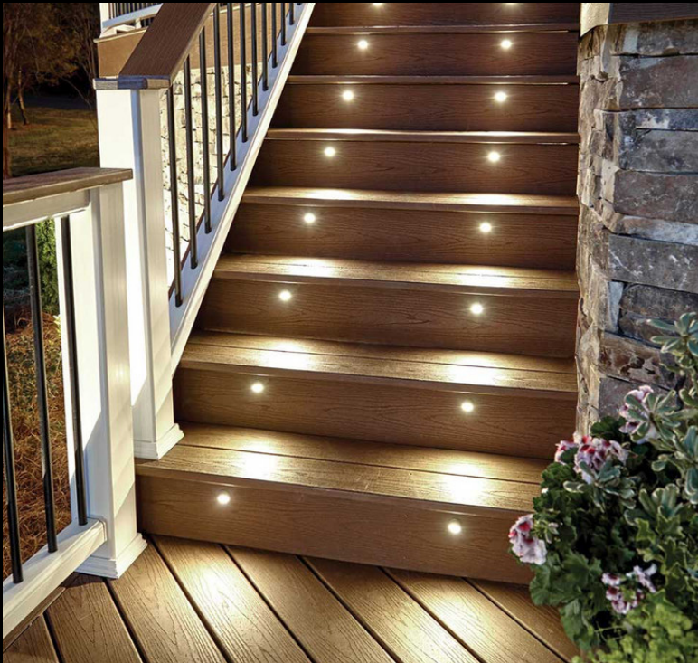
Deck Stair Lights
