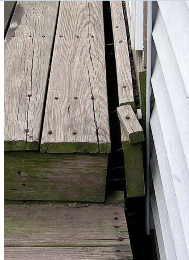
Nails alone don't do the job. This small deck was assembled by driving nails through the back of the ledger into the joists' end grain prior to installation. Toenailed joist-to-ledger connections are more common but also likely to fail.
