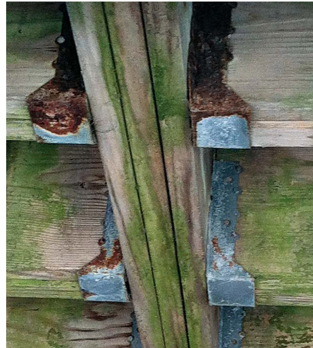
Use the right joist hangers. Although galvanized, the hangers on this seaside deck are rusty and nearing failure. Regular inspection of hardware is a good idea.
