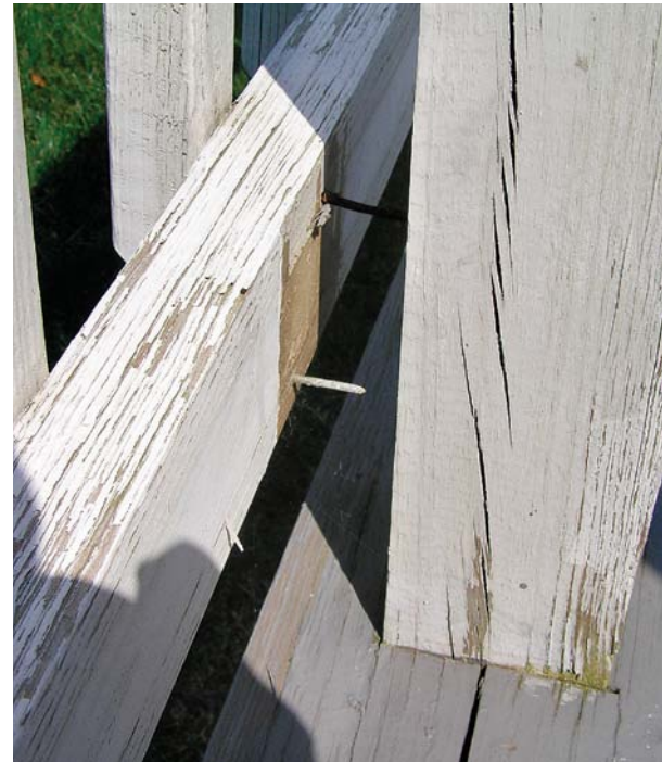
Don't rely on nails. This railing was just nailed to the outside of the posts. The nails eventually withdrew, and the railing pulled away.
