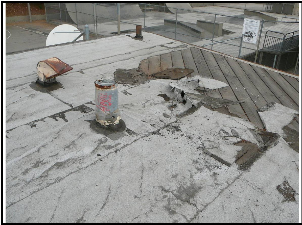
Photograph 7: View of the asbestos- containing roofing mastic material located on the roof of the Community Building.
