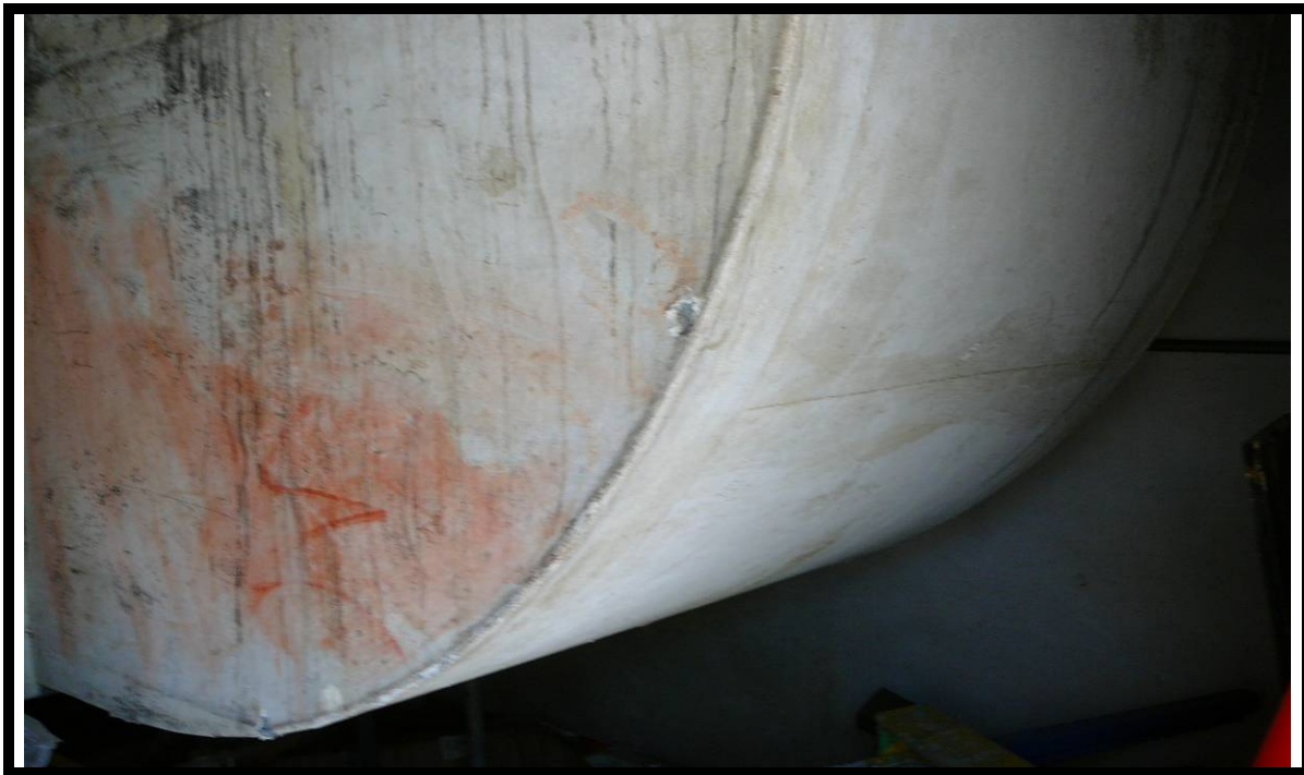
Photograph 3: View of the asbestos containing insulation material located on the HVAC ducting in the mechanical room of the Community Building.
