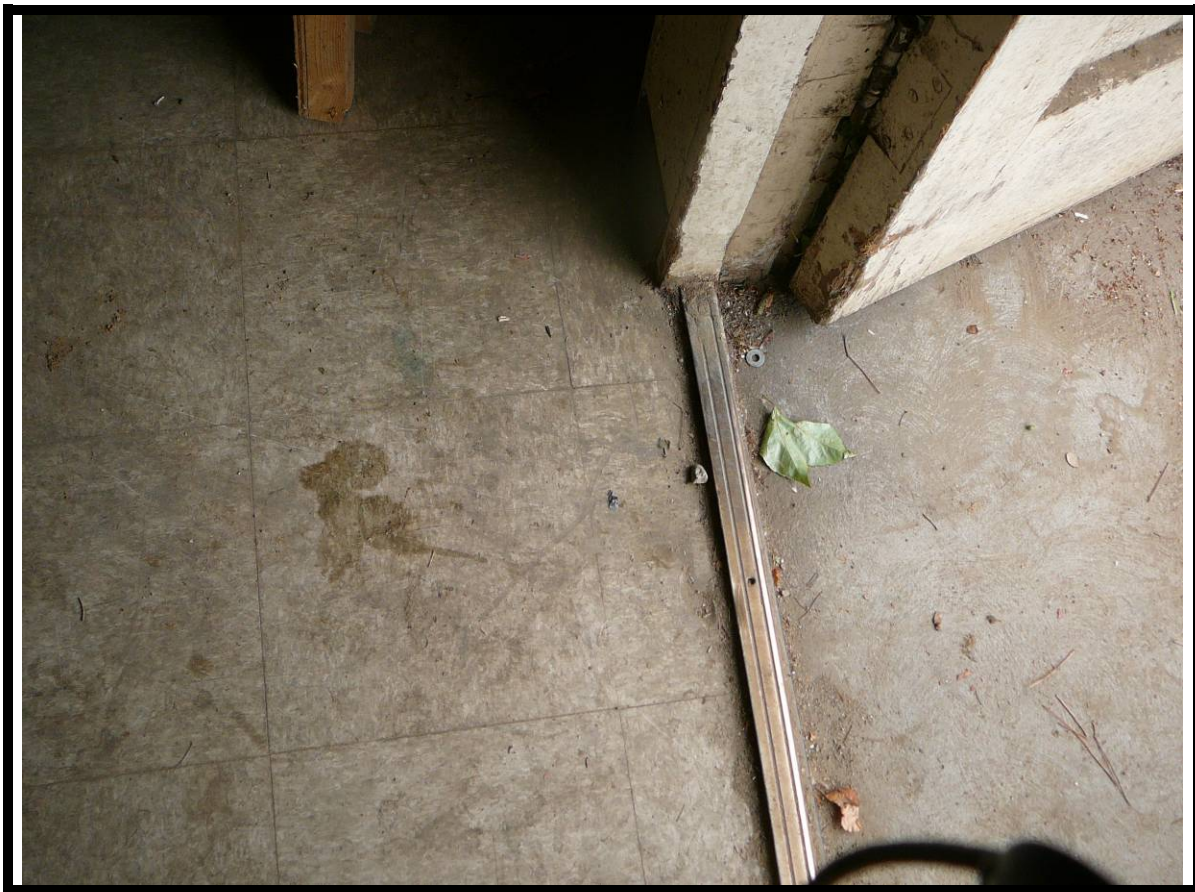
Photograph 2: View of the non-asbestos containing 12-inch by 12-inch vinyl floor tiles located in the auditorium and craft room of the Community Building.
