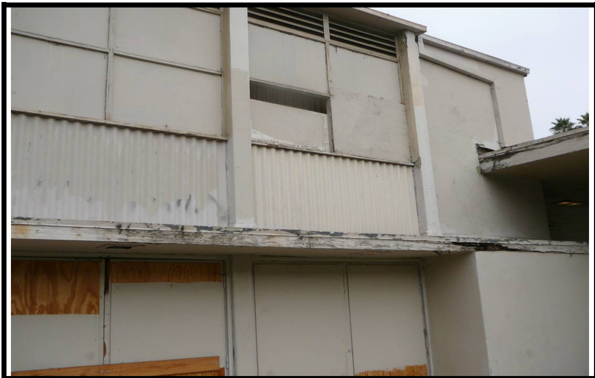
Photograph 6: View of the corrugated asbestos cement board material located on the exterior of the Community Building.
