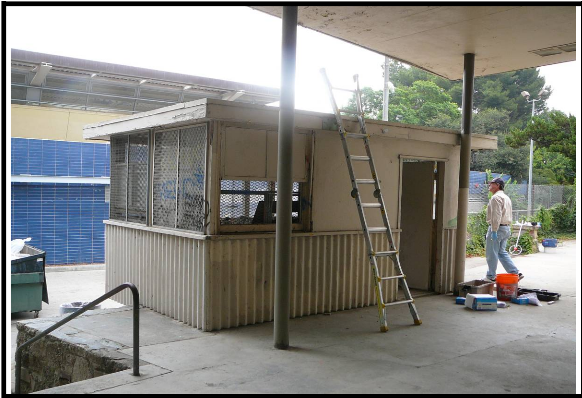
Photograph 5: View of the corrugated asbestos cement board material located on the lower section of the "office" structure at the Community Building.
