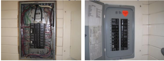
(laundry room – both sub panels)
