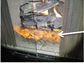
(primary bedroom) (Carbon monoxide concern)
