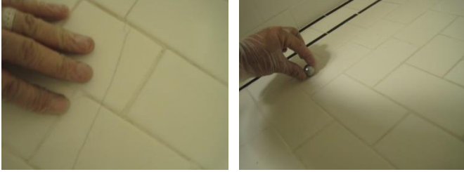
(hollow sounding tiles, cracks)
