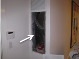
(the return air is outside the bedroom)
