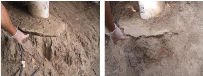
(this is building support for the guest house – soil support is very important here)
