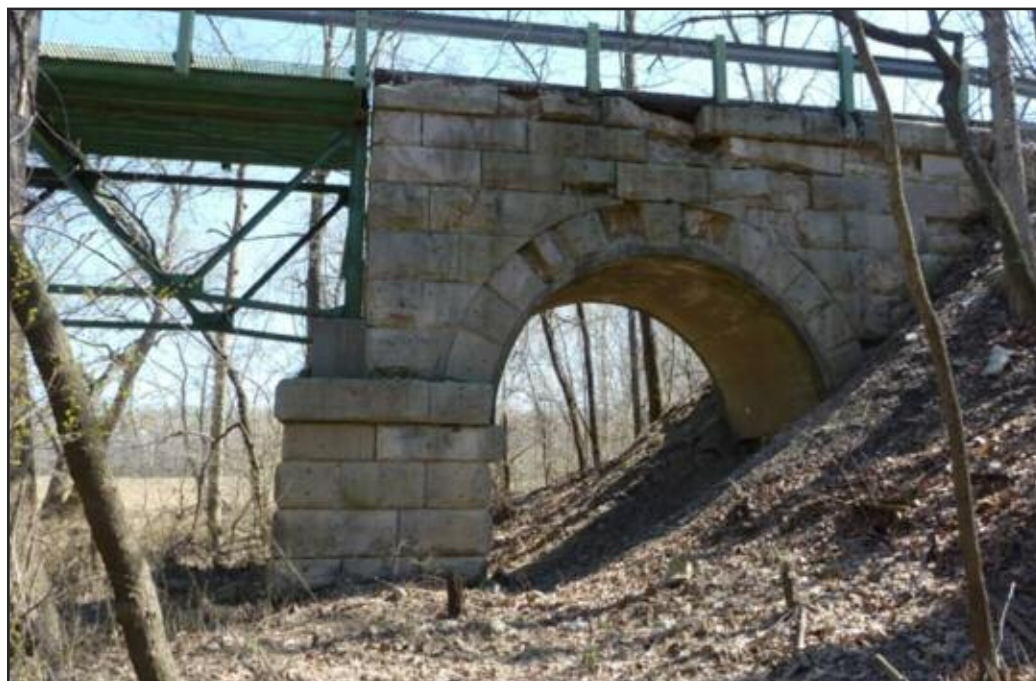
-Photo provided by the Indiana Division of Historic Preservation and Archaeology Martin County Bridge #58, located on Brickyard Road over Boggs Creek just north of Highway 50, circa 1890/1910, has a Warren deck that was built in about 1910 with limestone arch supports that were built in about 1890.
