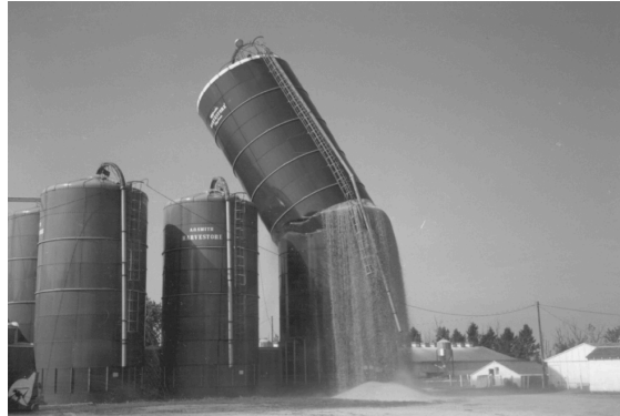
Figure 3.10. Example of silo failure.
