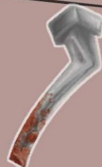
RUSTY PIPE: Old pipe, found in the third floor bathroom.
