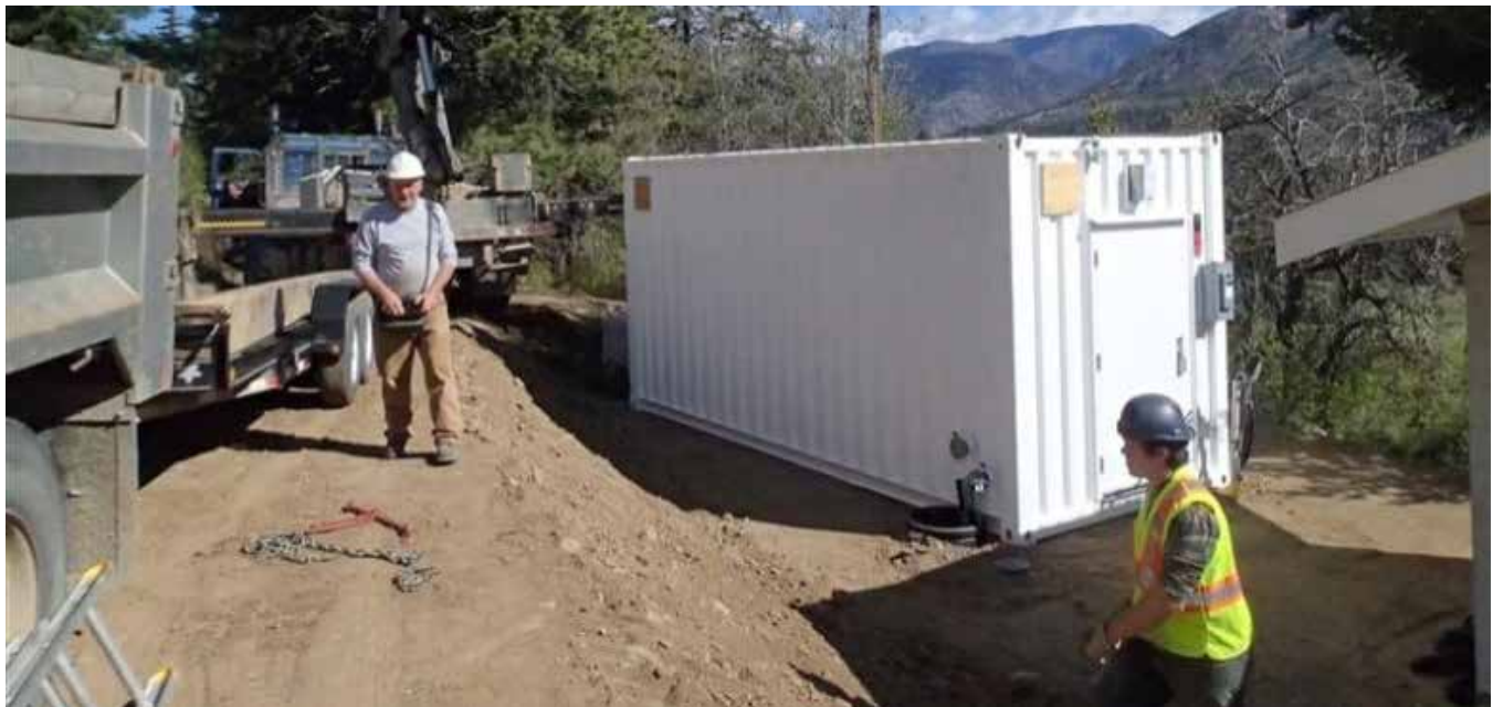
▲ A small, mobile water treatment plant is lowered into place on Lytton First Nation in 2019, helping end years of drinking water advisories. (RES'EAU-WaterNET)
