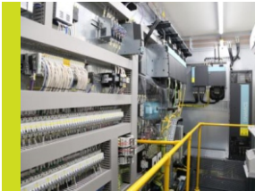
Port Equipment Electrical Room
