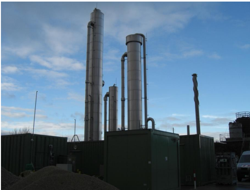
Fig. I: Biogas upgrading plant, Maihingen
