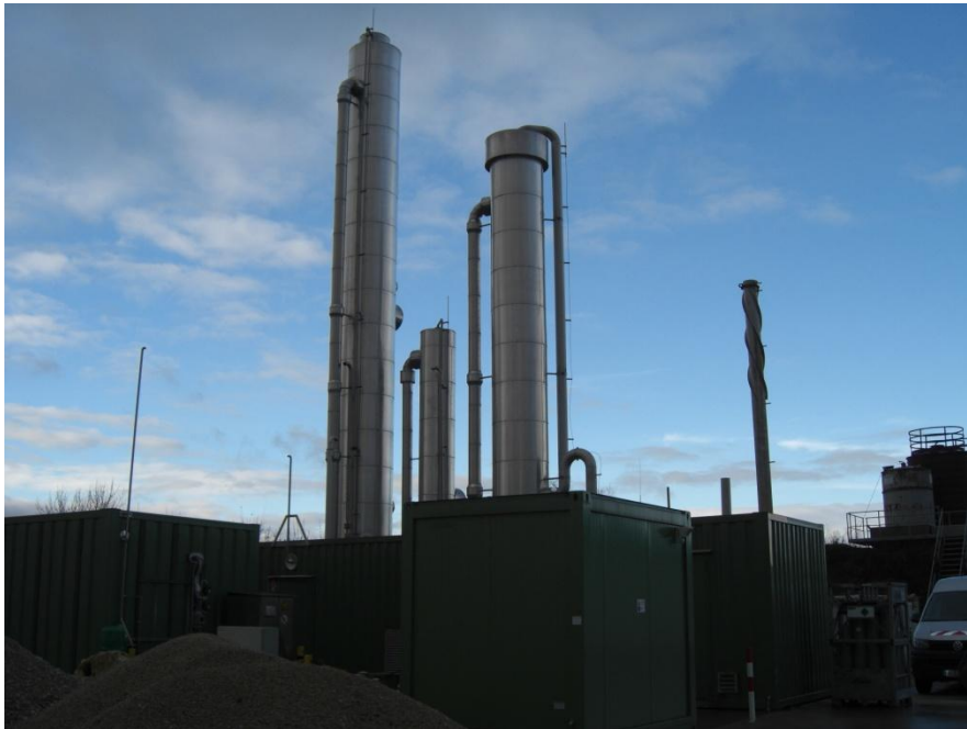
Fig. 2: Biogas upgrading plant, Maihingen (Source: Authors own)
