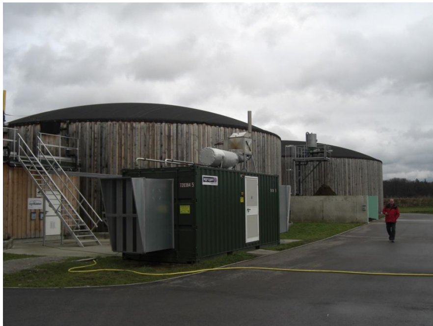
Fig. 3: Biogas plant at Triesdorf showing the two anaerobic digestion tanks and Combined Heat and Power unit (Source: Authors own)
