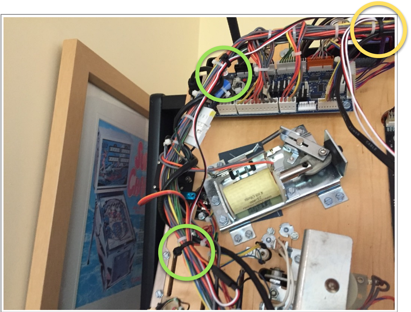
LHS Cable Routing
