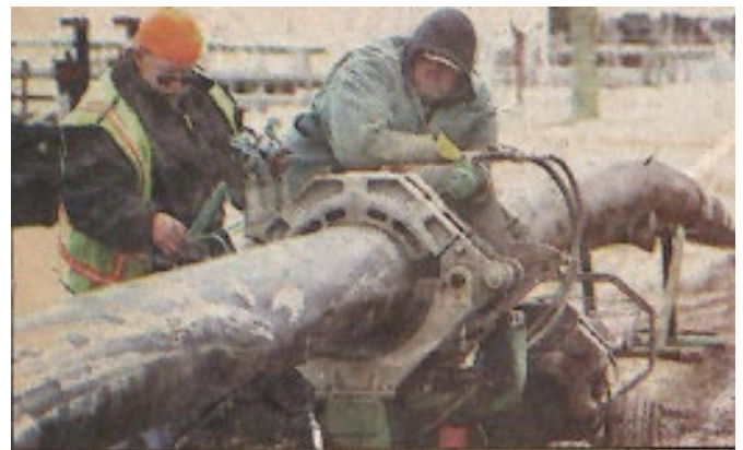
By TONY PITTS, Times Herald LINES GOING IN: Denny Howe of Mecosta, left, and J.R. Lucas of Garden seal a plastic water main pipe Friday as part of a project to supply city water to Harsens Island.
