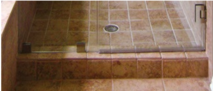
Increased likelihood of leaks.
