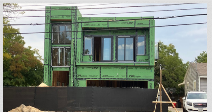
Example that would be out of building code compliance for a permit issued after Oct. 12, 2022.
