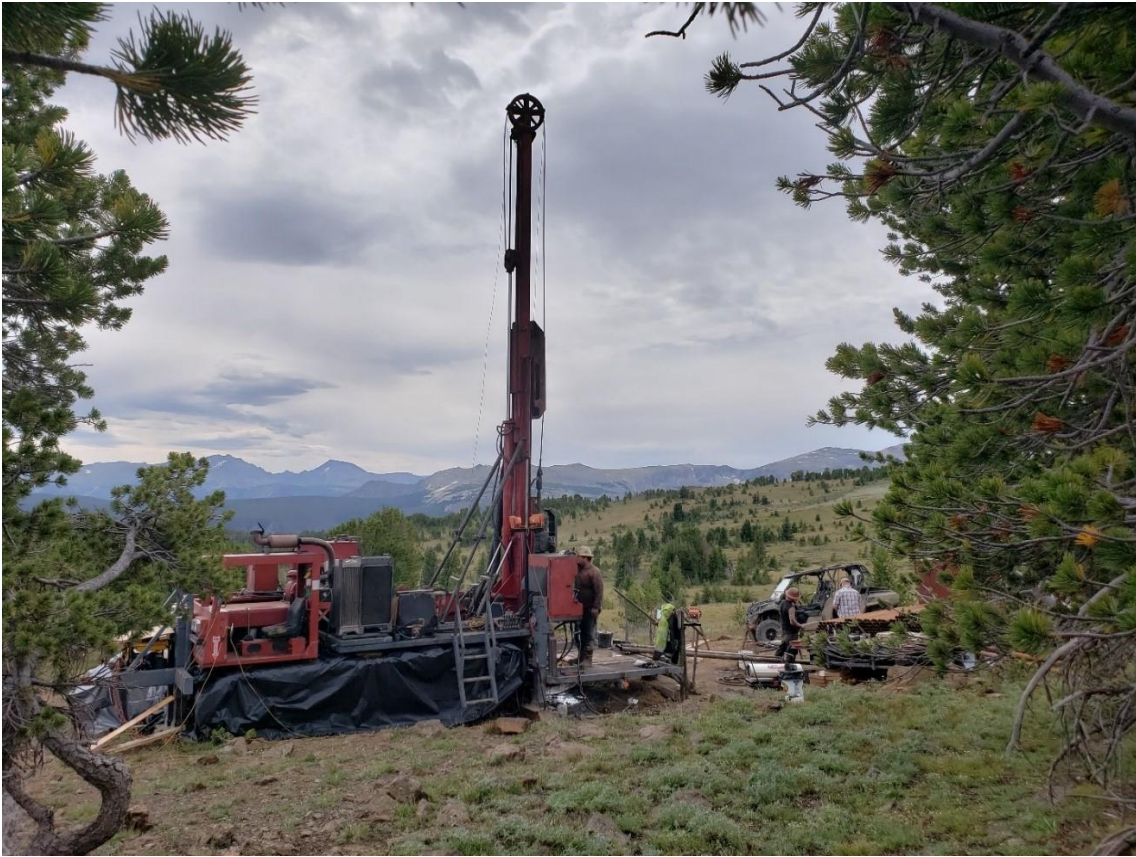
Figure 35. Drill rig on core Hole IM-2019-1 at the HGR target in 2019 (Photo by J. Modroo).
