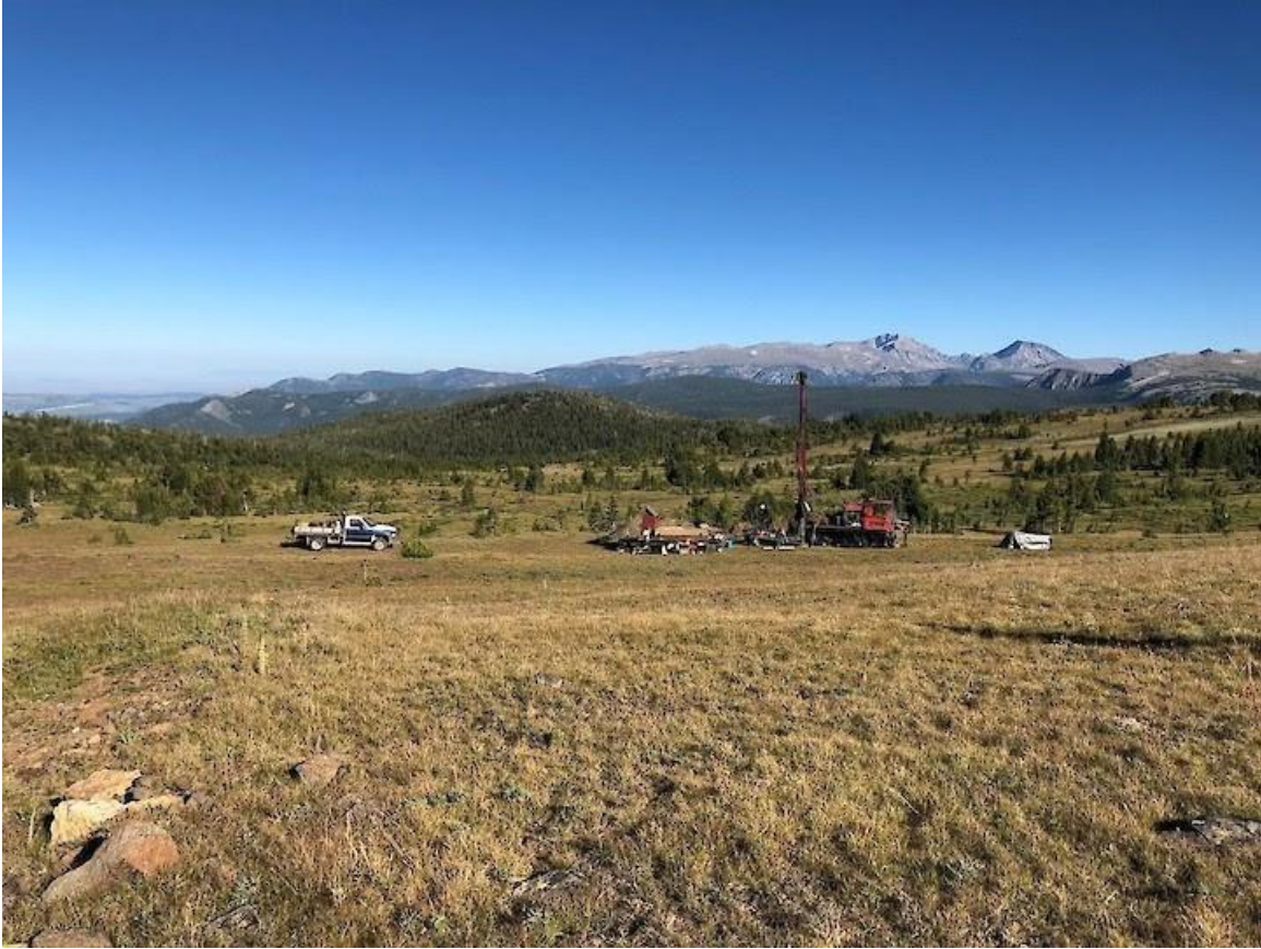
Figure 54. Photograph showing drilling in progress at the HGR deposit area during Group Ten's 2019 exploration program (Source: Group Ten News Release; September 25, 2019).
