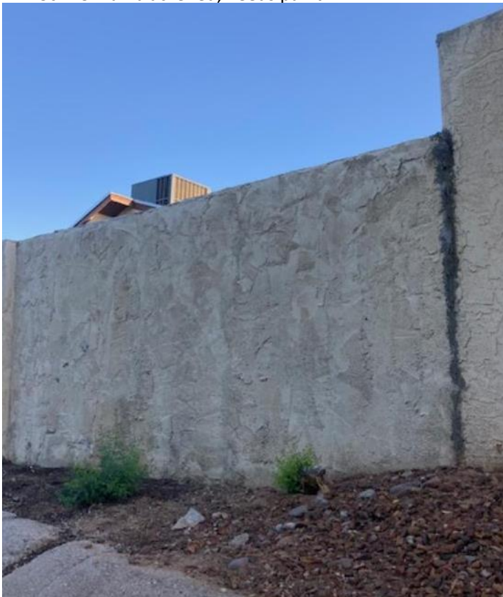
Lot #49 wall blackened, needs paint
