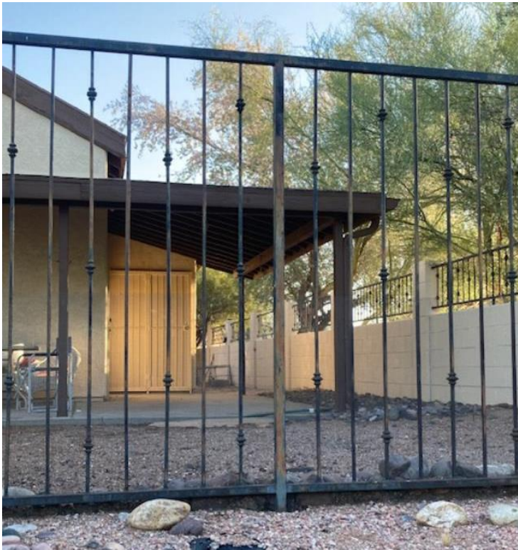
Lot #54 (wrought iron gate oxidized & rusted)
