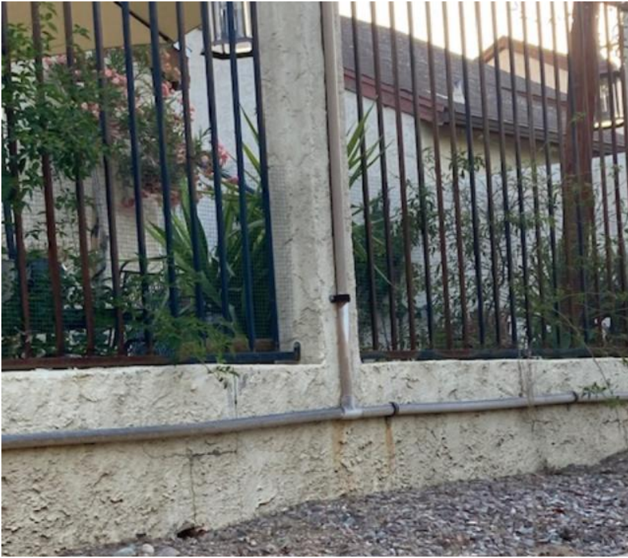
Lot #46 paint wall and pipes going along wall, paint fence oxidated & rusted
