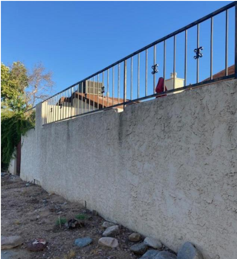
Lot #40 blackened, wrought iron oxidized & rusted
