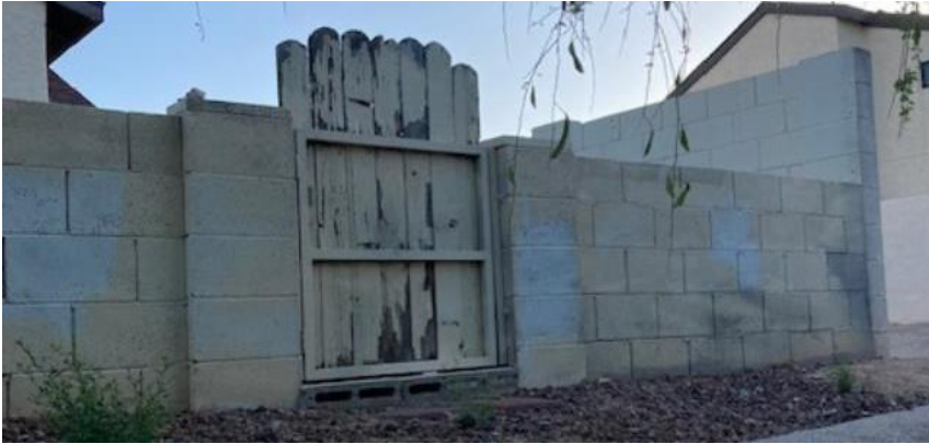
Lot #50 gate and wall need painting
