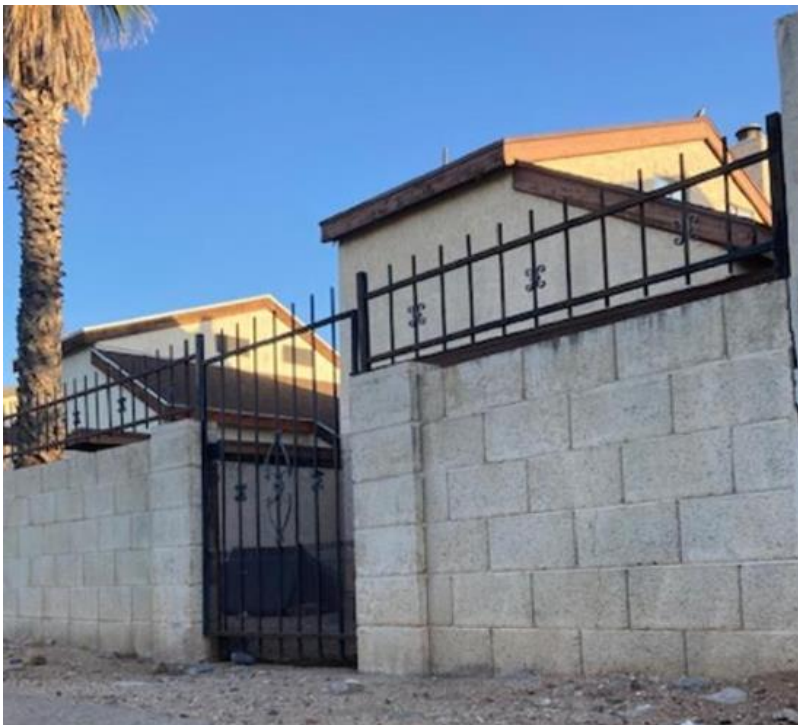
brick blackened, rust stains, wrought iron oxidated & rust
