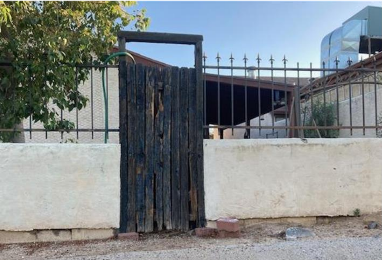
Lot #45 wall Needs paint, also wrought iron oxidized & rusted
