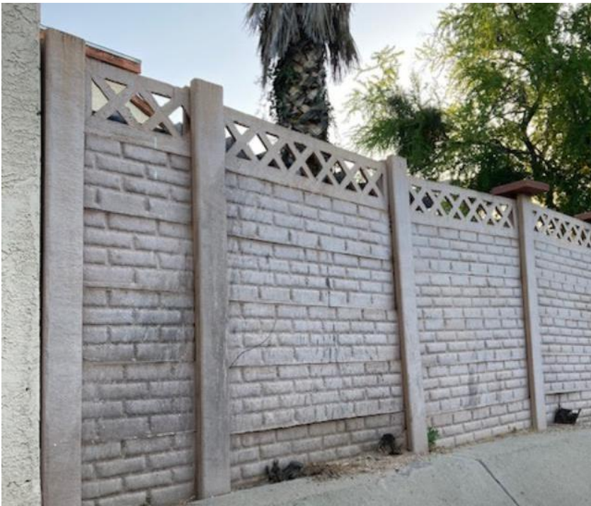
Lot #35 Needs paint
