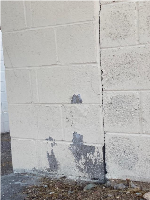
Lot #37 paint missing in chunks & splotches
