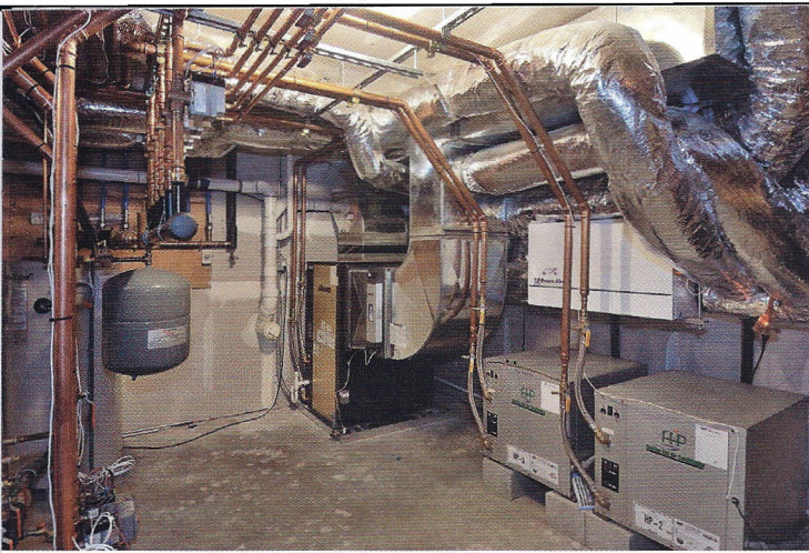
Florida Heat Pump units are tied into the geothermal system for the Kennedy home in a basement mechanical room showing extensive use of copper piping. (Photos provided by Jim Fuhrmann of Jim Fuhrmann & Associates)
