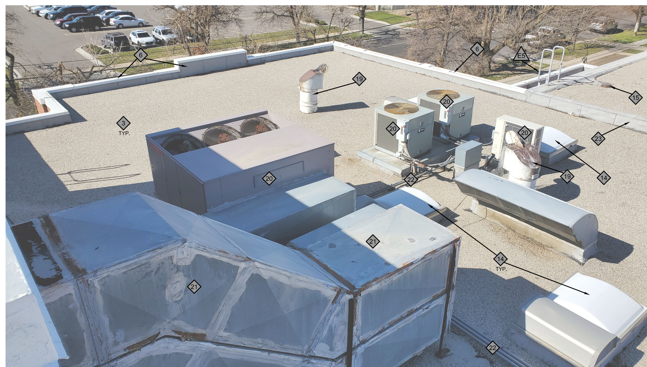
PHOTO: WEST MIDDLE ROOF EQUIPMENT
