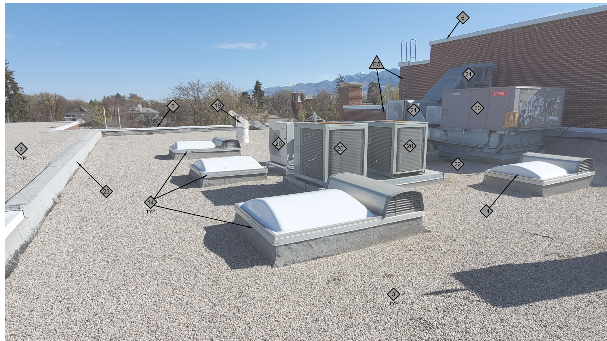
PHOTO: WEST MIDDLE ROOF EQUIPMENT
