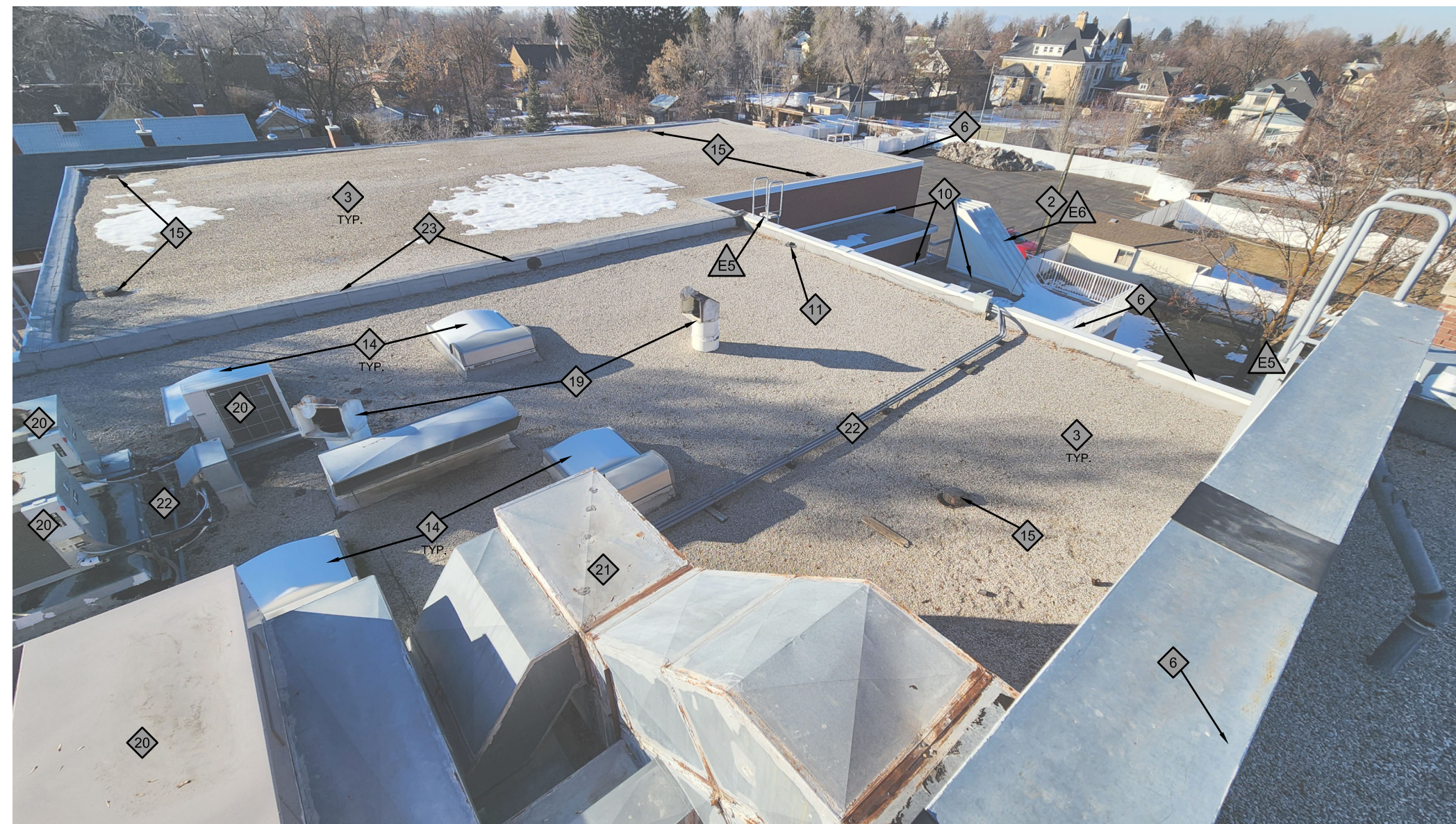
PHOTO: WEST MIDDLE ROOF EQUIPMENT
