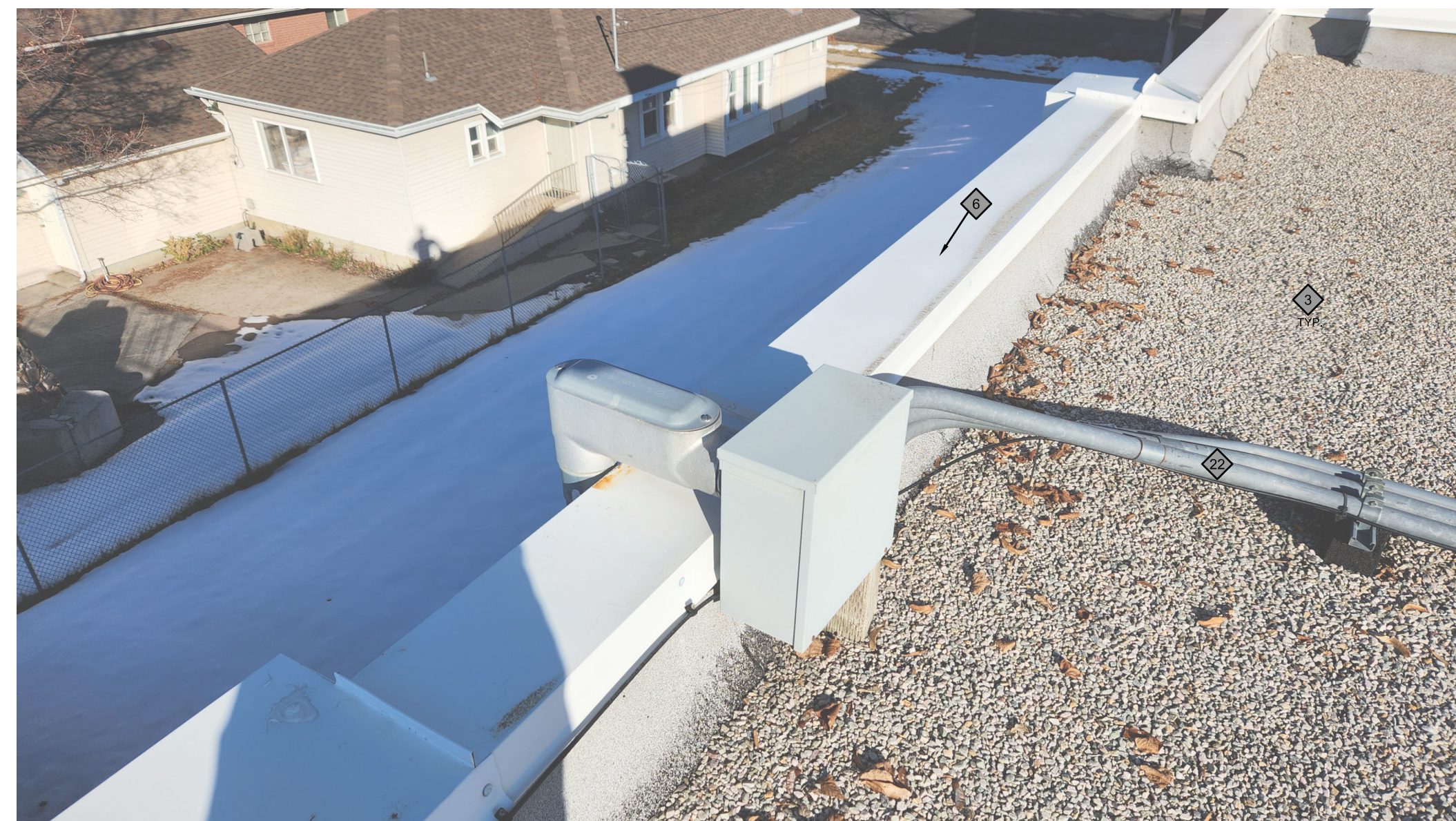
PHOTO: ELECTRICAL BOX
