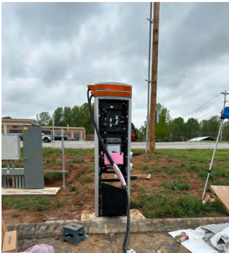
Fast Chargers Arriving at Ascension Saint Thomas River Park Hospital
