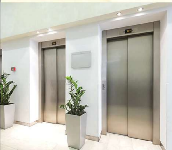
Lift & Common Area with Power Back-up
