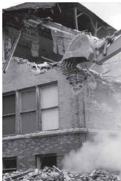
Washington School was torn down with a 9050B Case Track backhoe. Area residents took home bricks as mementos of the neighborhood school.
