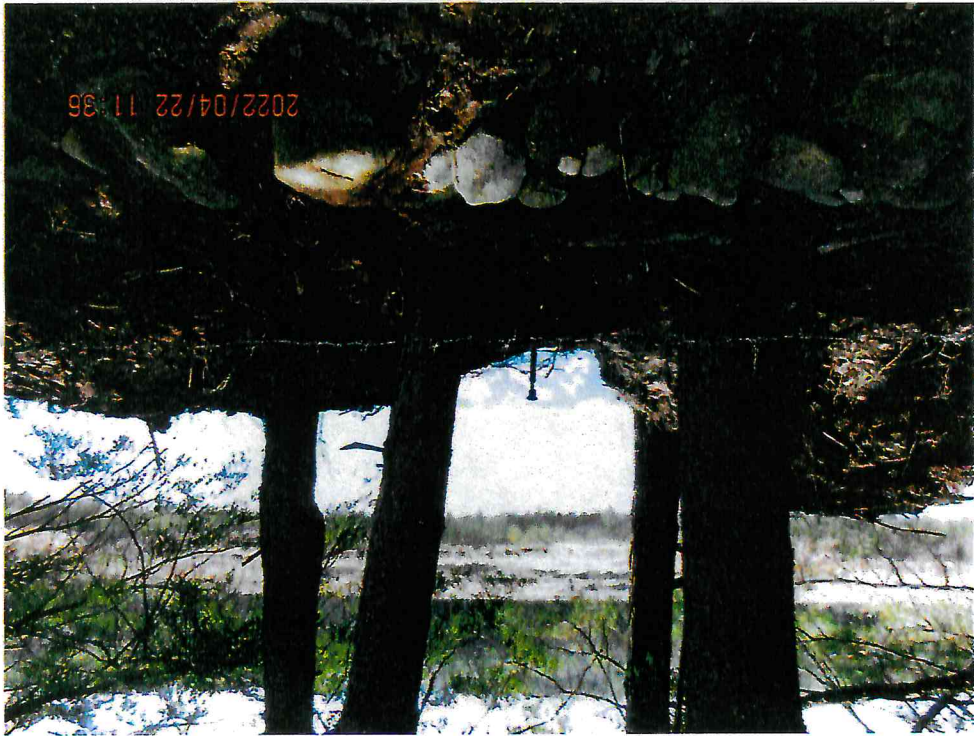
Photo 3. Debris on embankment upstream slope.
