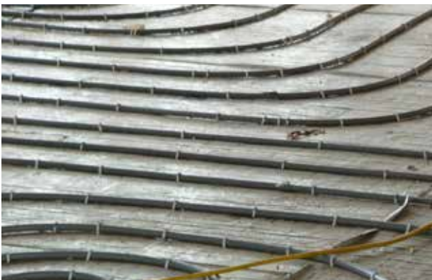
Underfloor heating being laid in a public building in Somerset. Underfloor heating is often a feature of low-carbon homes and buildings.
