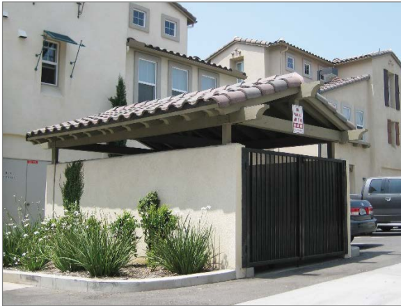
Enclosing trash facilities in structures that blend in with the architecture of the building helps minimize the appearance of these uses.
