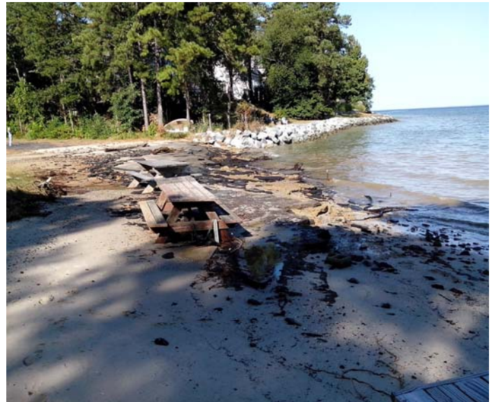
Erosion of beach and exposure of asphalt
