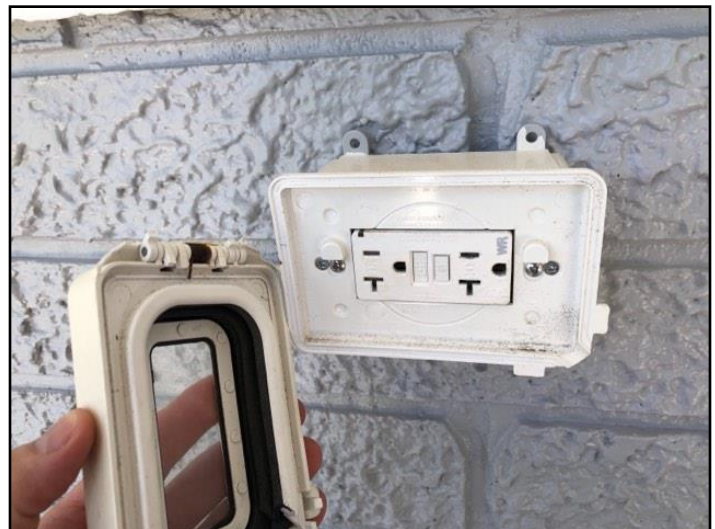
Cover broken at front entrance
