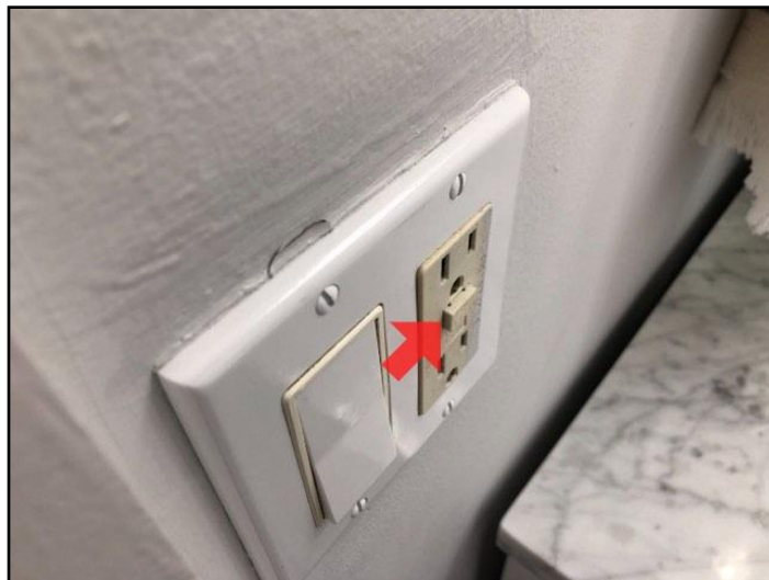
Failing GFCI receptacle
