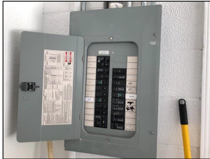
Breakers not properly labeled
