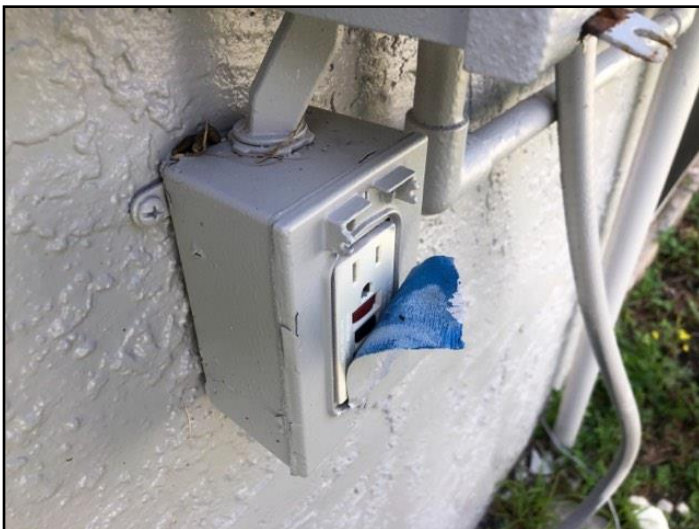
Cover missing beside pool pump
