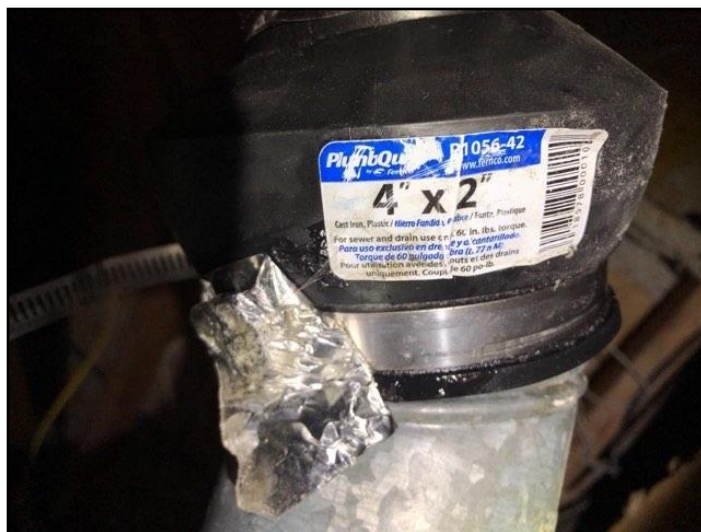
Wrong connector for exhaust connection
