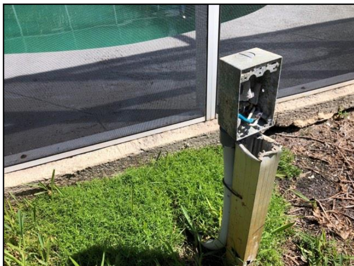
Light junction box corroded
