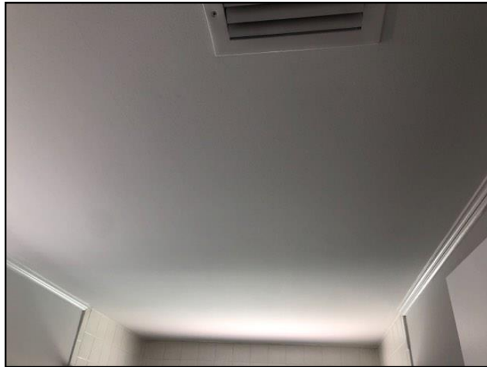
Exhaust fan not installed
