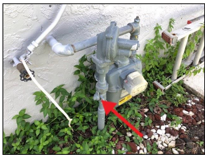
Main gas shutoff valve
