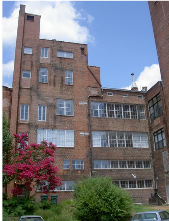
Windows: Original steel frame windows, with double pane transparent glass. Frames painted silver. New windows on the rear façade match frame color and pane size of original 6 over 6 windows.
