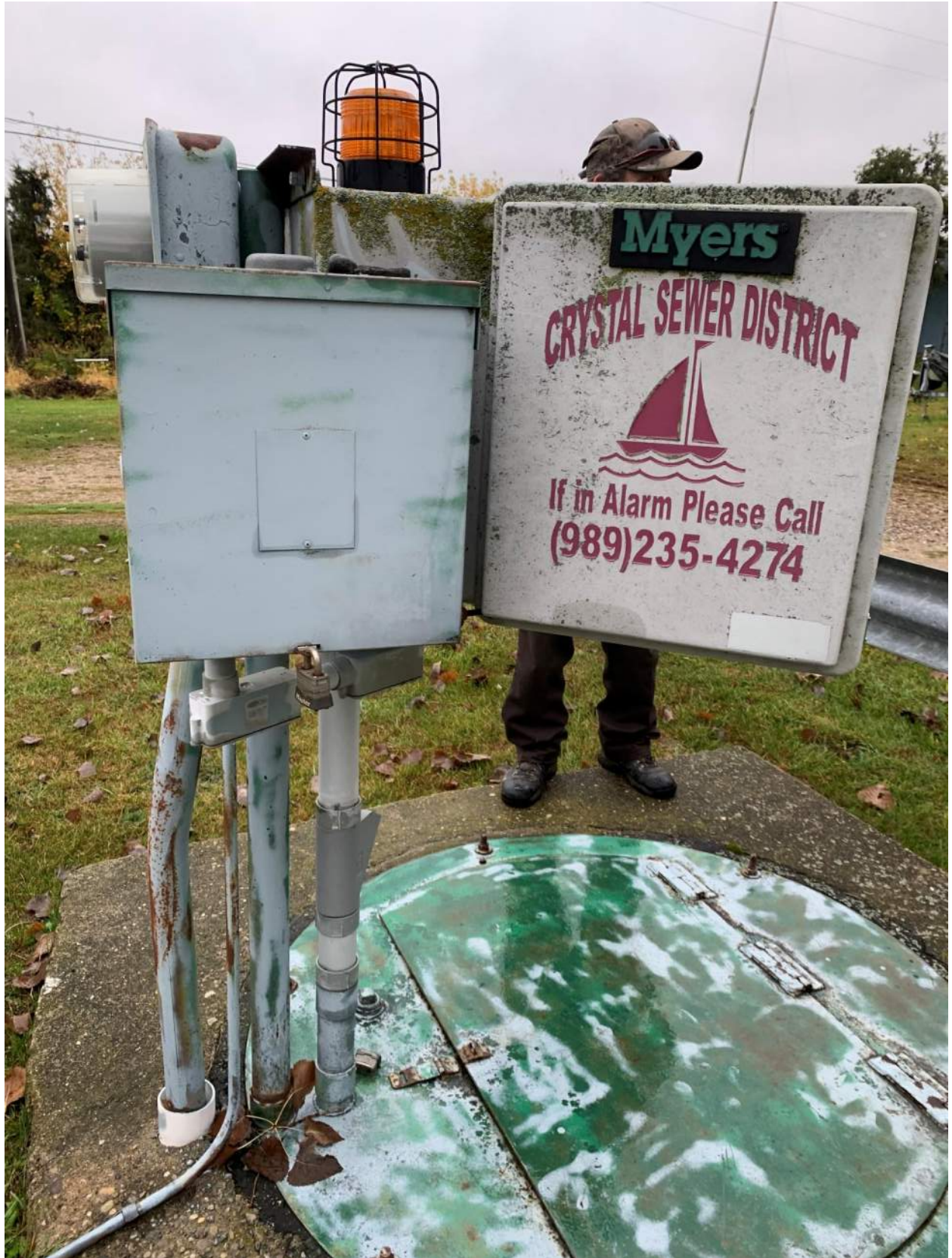
One of the Lift Stations to be Reconstructed
