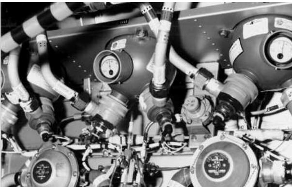
48f. REAR COMPARTMENT ENGINE FIRE EXTINGUISHER—CHECK
