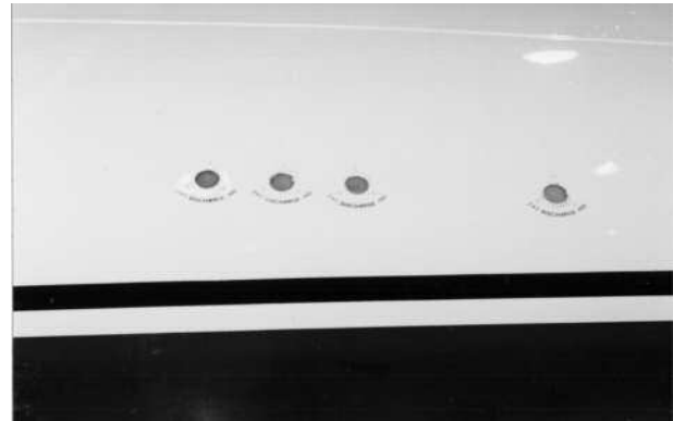
49. FIRE EXTINGUISHER FRANGIBLE DISCS—CHECK
