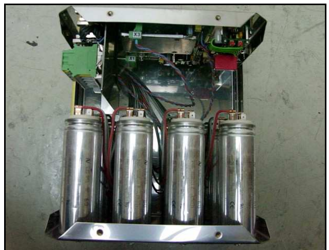
Fig. 4.8.3-2: Opened AC Control Box from Panda 30 upwards
