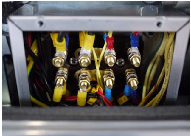
Fig. 3.3.5-6: Generator power terminal box
