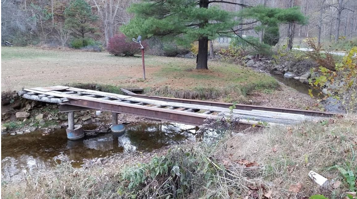
Figure 1: Poorly Designed Private Residential Bridge Before Bridge Home Program Replacement (Courtesy of WV VOAD)
