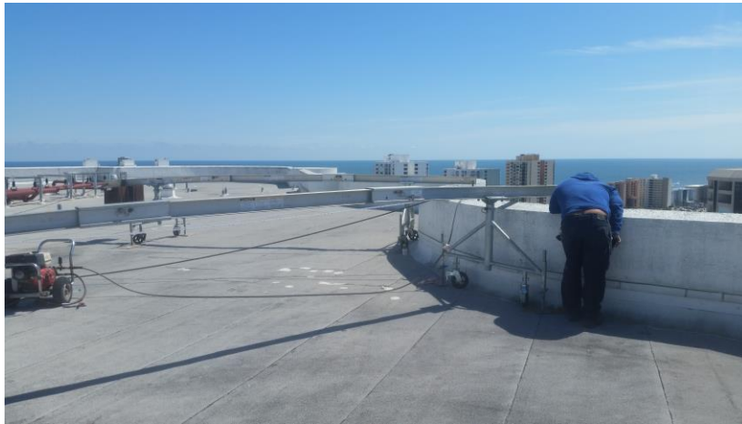
Roof Top Scaffolding Anchor System
