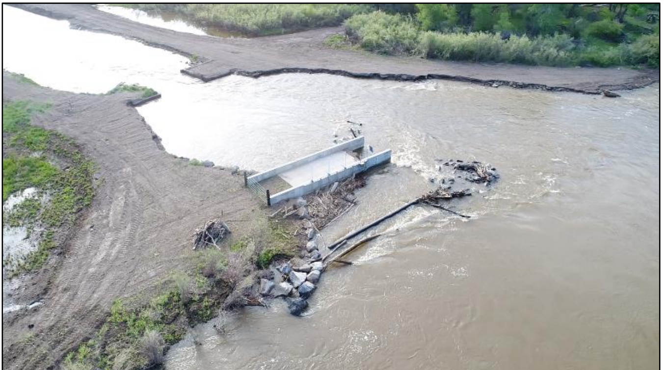
Aerial photograph of bank failure adjacent to recently installed headgate. Photo taken Spring 2019.
