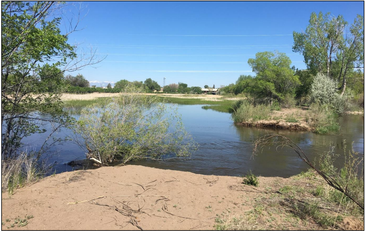
Failed levee north of diversion dam during Spring 2019 runoff
