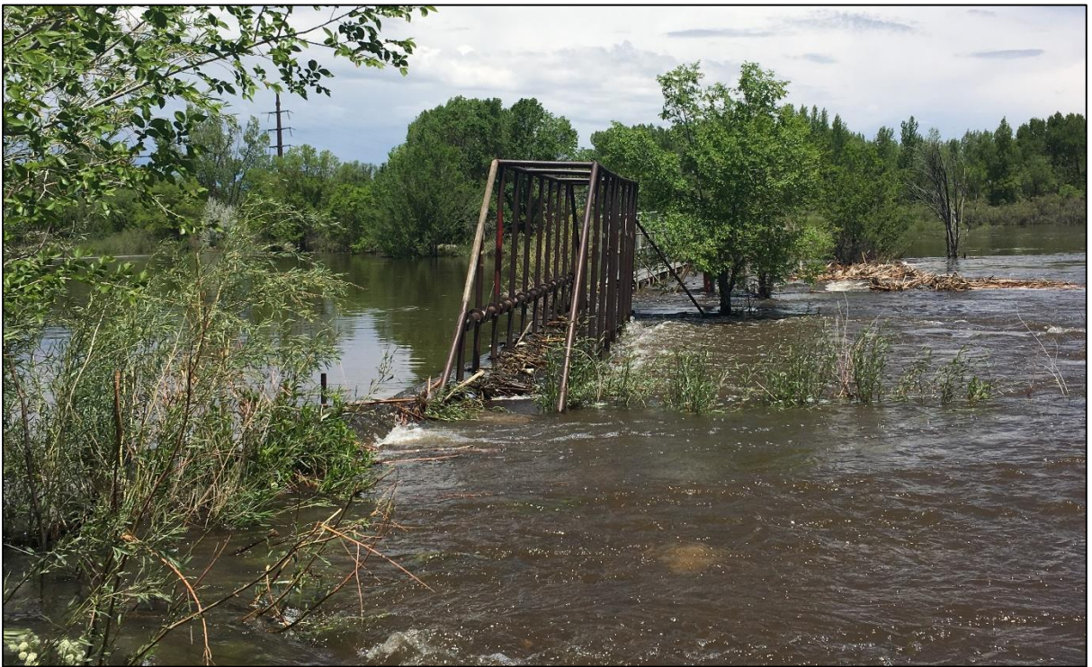
Flooded diversion dam during Spring 2019 runoff
