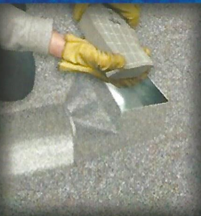
Wall registers are covered in order for air to escape only through leaks
