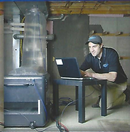
AeroSeal software allows the technician to accurately measure the duct leakage in your home
